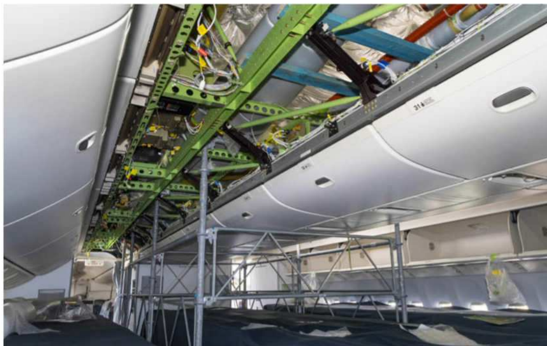
Images of VH-PPH's Wi-Fi installation. SETH JAWORSKI
